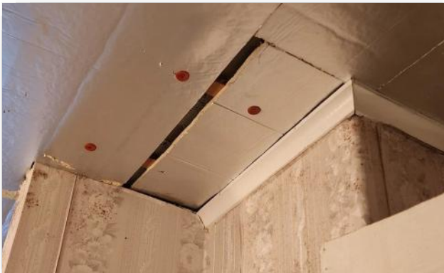
BEFORE HOME REPAIR EXAMPLE
